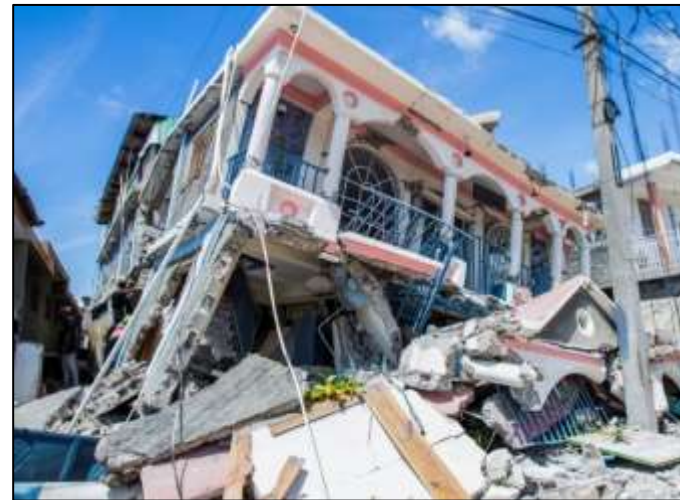
Damage caused by a 7.2 scale earthquake that hit the country of Haiti in August 2021.
